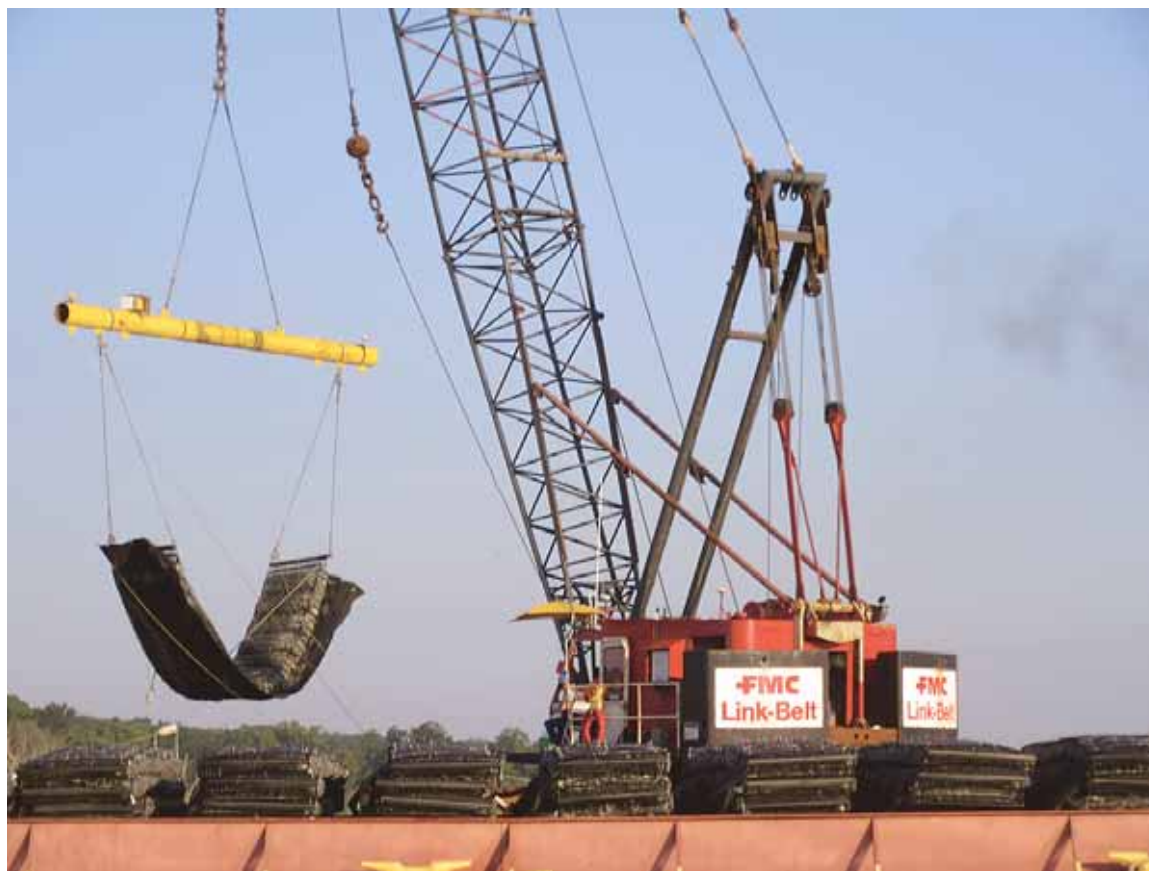
A crane lowers a marine mattress into the river to support the breakwater.
